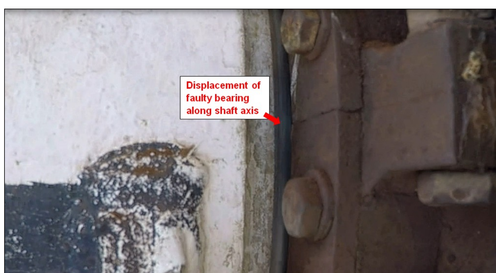
Figure 4: Bearing at west end of Dec shaft shows displacement of \pm 10 mm. Credit: P. Mey.
